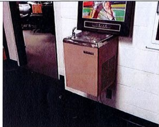
20. Non-compliant single ADA drinking fountain.
