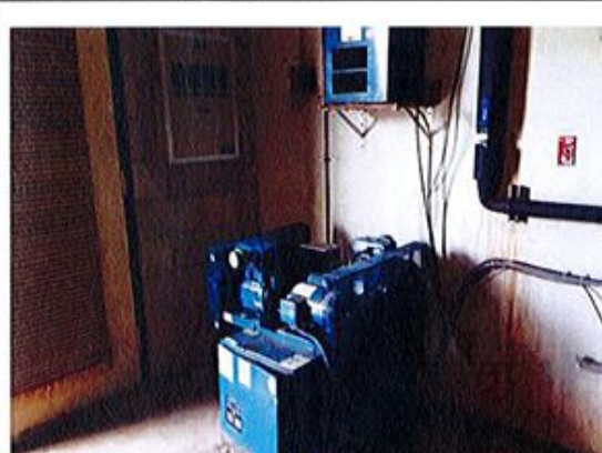
12. Mechanical room with moisture in walls.
