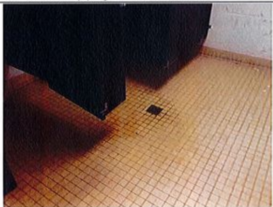
17. Drains clogged in unused restroom.
