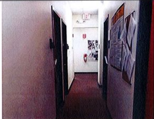
21. Corridor width not 48" ADA compliant.
