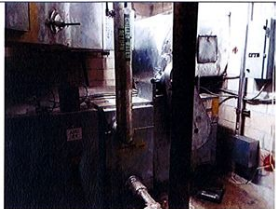
14. HVAC unit in mezzanine.
