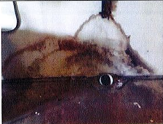
11. Drain in mechanical room with mold into gypsum board.
