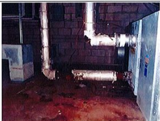
15. Corroded piping in mezzanine HVAC.
