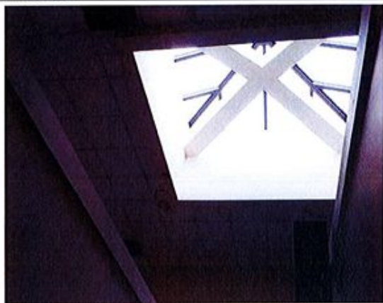
19. Apparent leaks in roofing around skylight.
