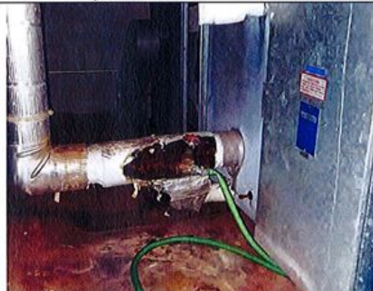
24. More corroded piping in HVAC mezzanine.
