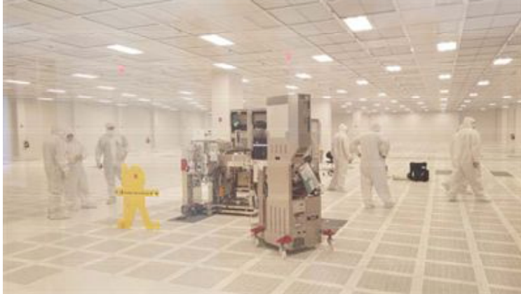
Front of Class 100 Cleanroom - 1 st Tool Placed - October 2017
